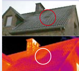
The infrared inspection locates missing insulation in the roof. This can now be repaired and further energy loss prevented.
