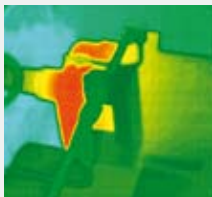
Motor: Bearing Problem
