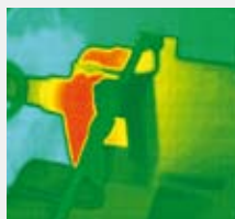
Motor: Bearing Problem
