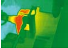
Motor: Bearing Problem
