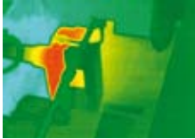
Motor: Bearing Problem
